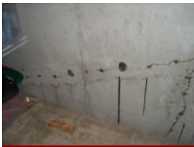
Prior Foundation Repair
