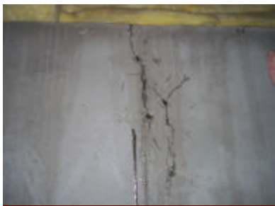
Prior Foundation Repair
